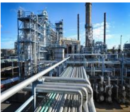
Oil, gas, and other infrastructure facilities
