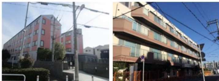
Renovation of the old company dormitory in Yagumohigashi-machi, Moriyuchi-shi (to be completed on Jan. 27, 2025)
