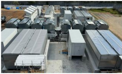
Container-type data centers under construction on the site of Ishikari Data Center
